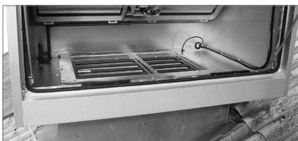
Fig. 33: Extract air filter installed in the unit
