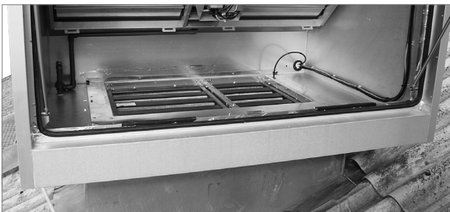
Fig. 28: Extract air filter installed in the unit
